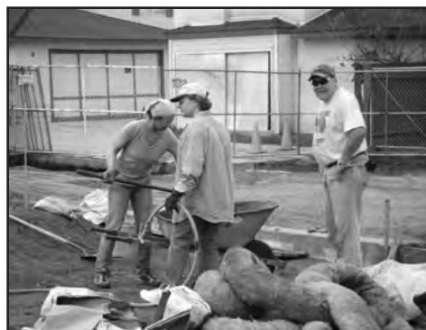
Heather West, Barbara Higgins and Lee Mercer mix cement at the building site.
