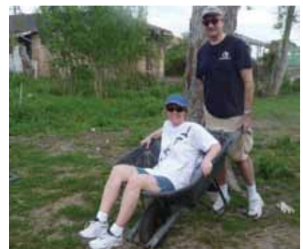
Precious cargo! Jack Krecek gives his wife Fran a lift on the building site
