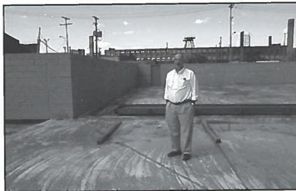
Al Walcutt in the middle of MPC's new building construction site. Behind him is where the new plating line will be located.
